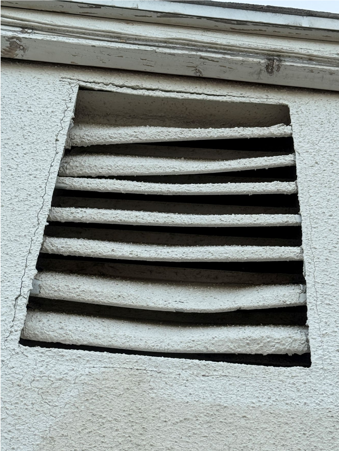
Figure 5 – Gable vent exclusion with netting
